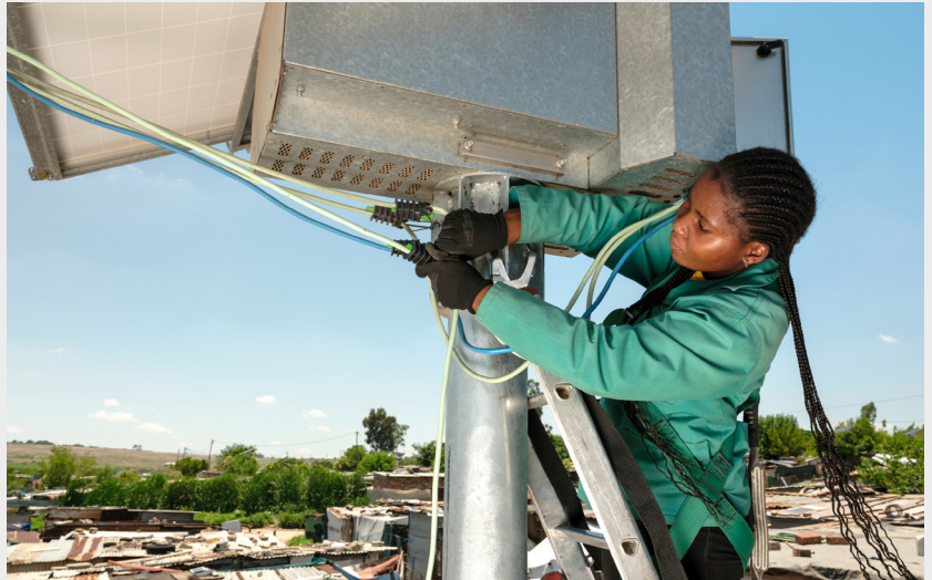
In South Africa, new solar installations are bringing 3500 households access to electricity, as well as employment.
