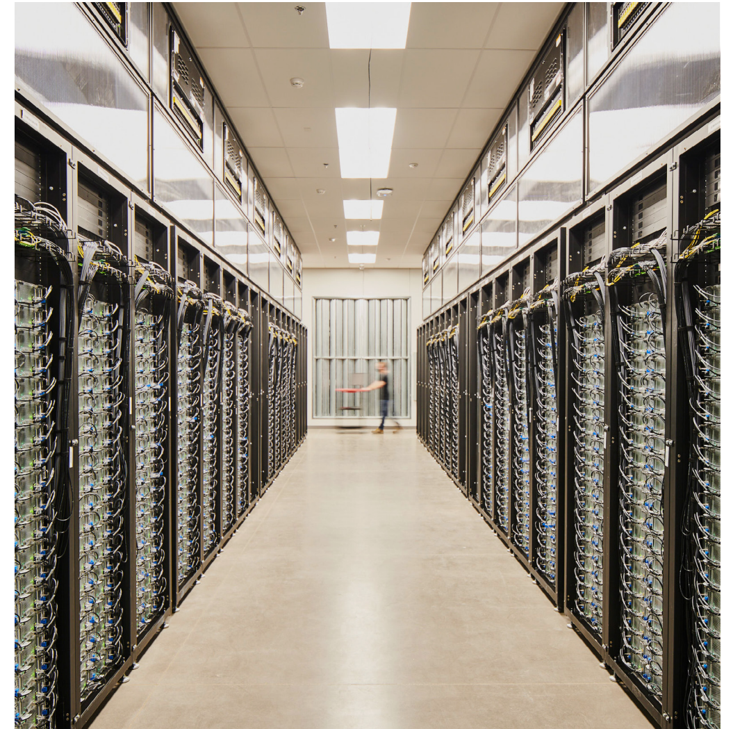
Apple's Reno data center, opened in 2012, takes advantage of the mild climate by cooling its servers with outside air whenever possible.
