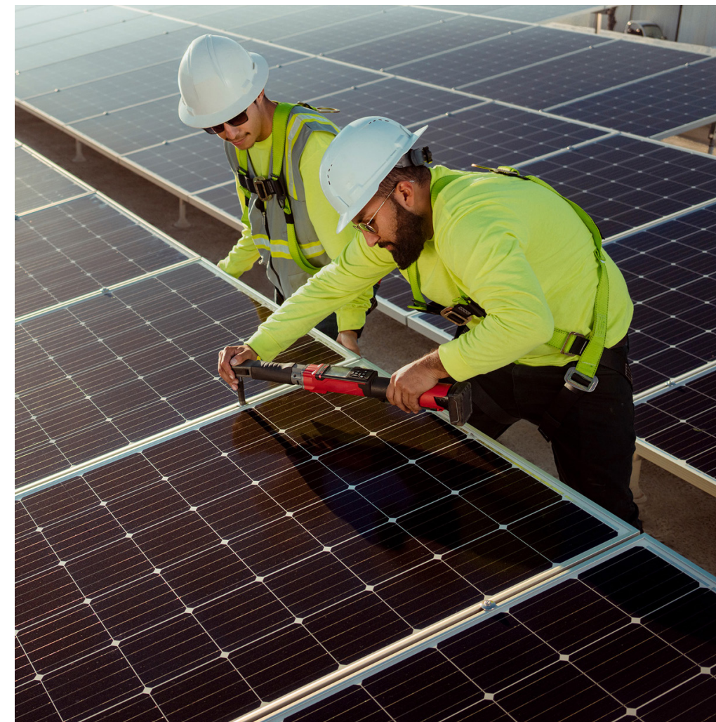
Technicians from Simmitri perform maintenance on solar panels installed at Bench-Tek Solutions in Santa Clara, California. Both companies are alumni of the Apple Impact Accelerator.
