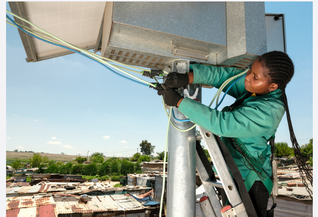
Power for Impact is expanding access to clean, affordable power in different parts of the world. Apple will continue to focus on uplifting communities as it pursues its environmental goals.
