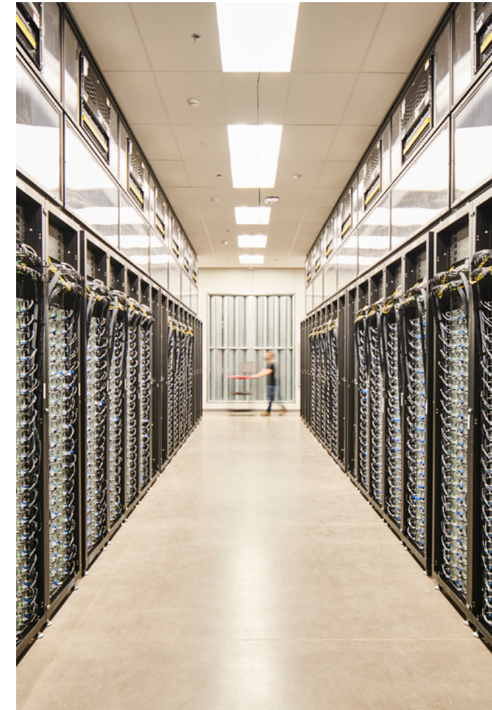
Apple's Reno data centre, opened in 2012, takes advantage of the mild climate by cooling its servers with outside air whenever possible.
